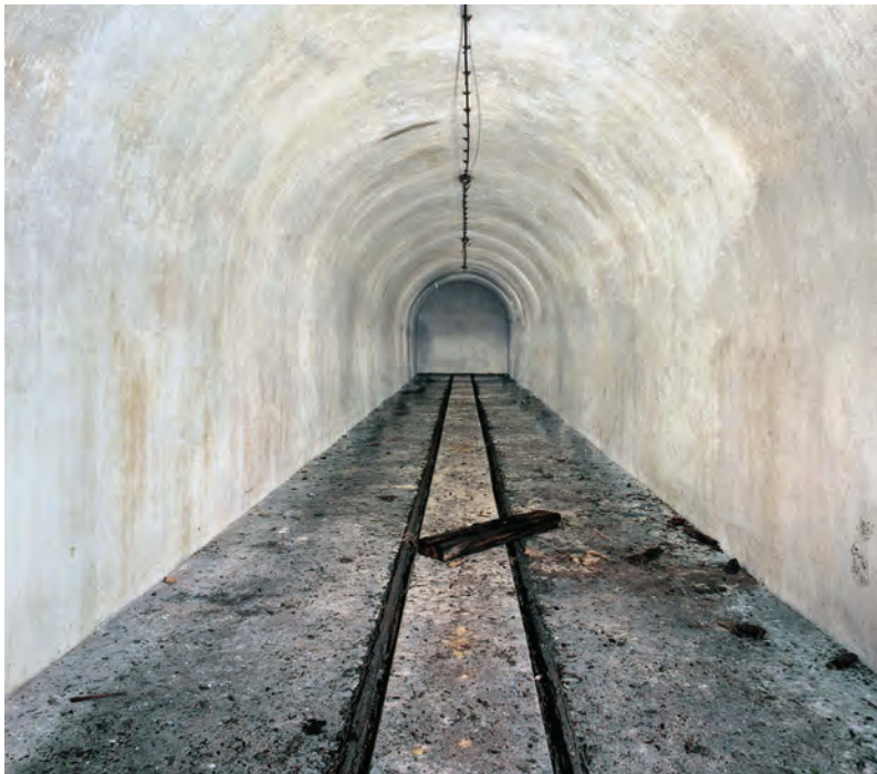
A storage chamber in Ho 5 on the east side of Water Lane. The concrete-lined chamber is clean and dry with 60cm railway track embedded in the floor. The tunnel leading to it is wet and difficult to access. It was cut through soft diorite rock and was timber-propped throughout. The props have all collapsed leaving deep 'sludge' on the floor. For a picture see previous page. The tunnel was used as a fuel store and electricity generating station.
